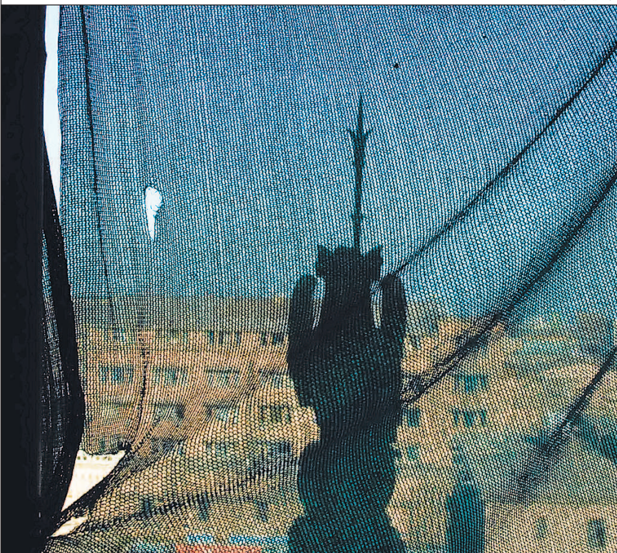
STANDING TALL: Restoration work of Chhatrapati Shivaji Terminus is on in full swing
